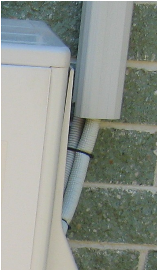
Figure 43 Ducting open at the end
