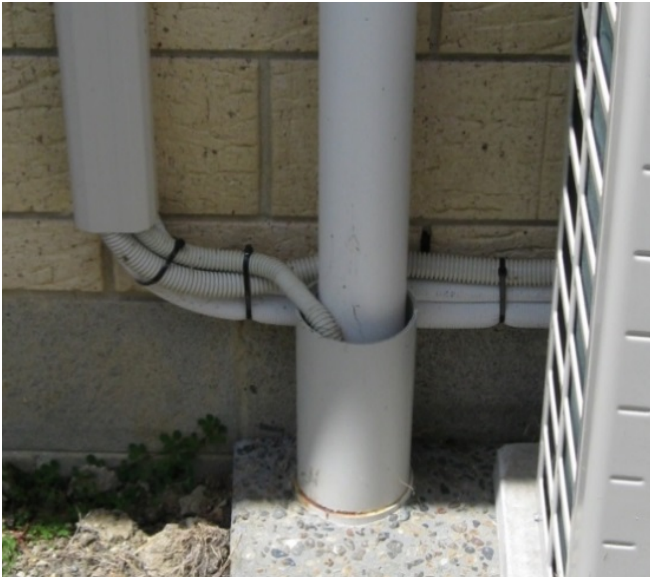
Figure 45 Drainage pipe directed into a drain
