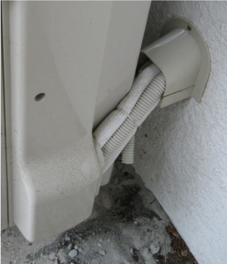
Figure 44 Draining on to concrete path – very typical
