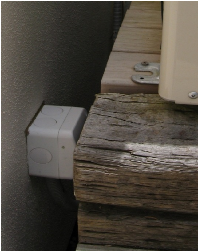
Figure 47 Placement of isolator switch means it is impossible to use
