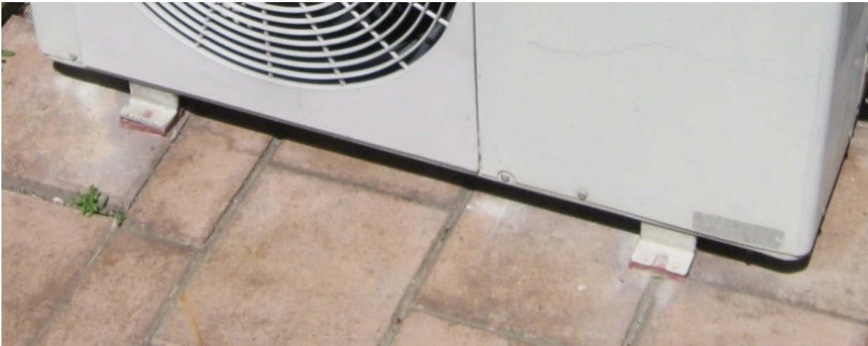
Figure 41 Very little clearance under the unit
