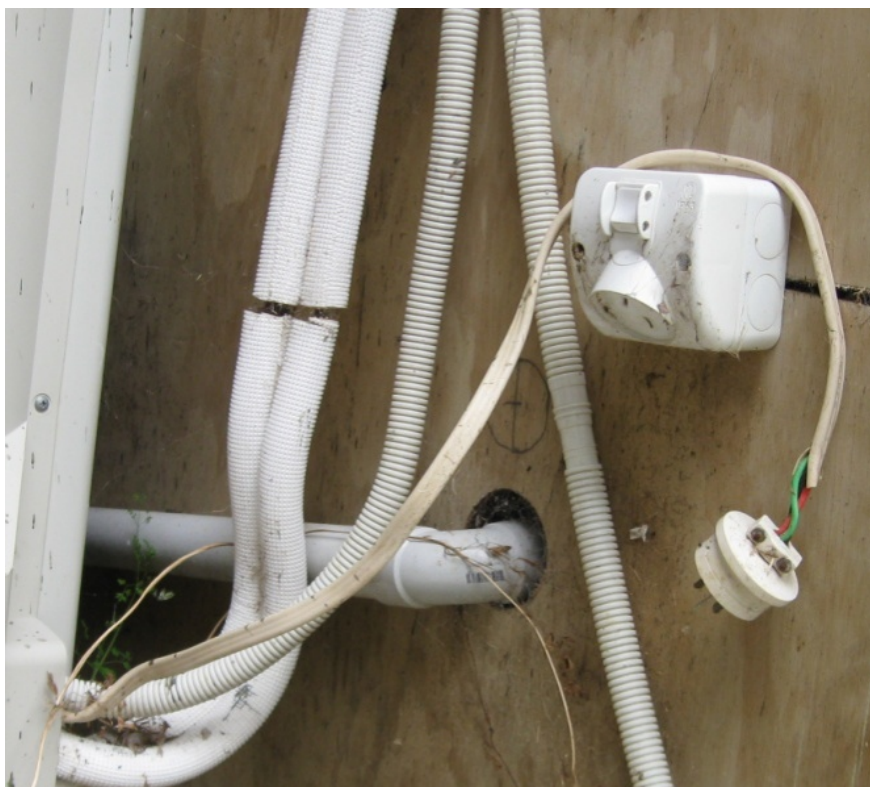
Figure 46 One of the worst examples of wiring found
