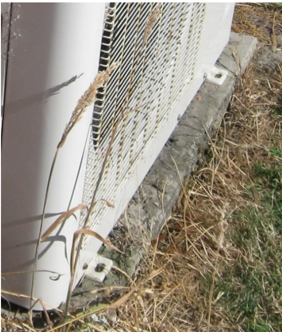
Figure 42 No clearance under the unit
